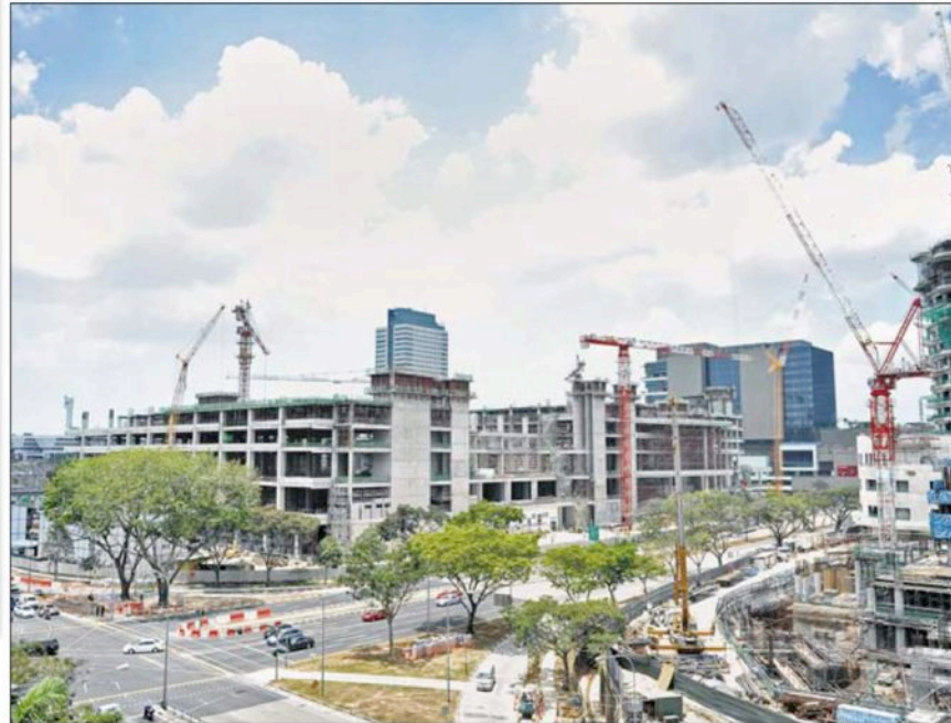
Big Box, which has 400,000 sq ft of retail and dining space, will be run by a single operator, TT International, under EDB's Warehouse Retail Scheme. ST PHOTO: MATTHIAS HO
